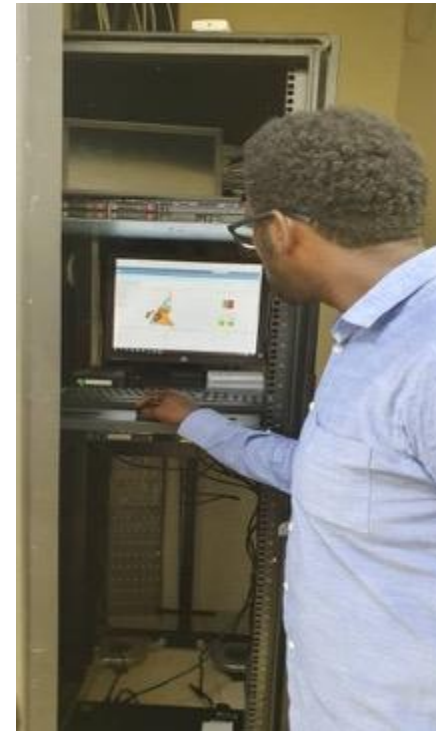
Installation completed successfully at server 1
